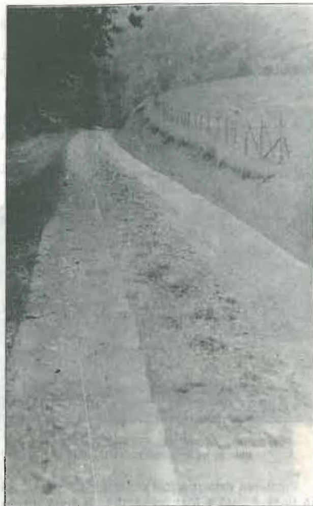
Foto 5. Vedere de ansamblu a tronsoanelor la doi ani după execuție. (General view of the roads two years after they had been put into execution).
